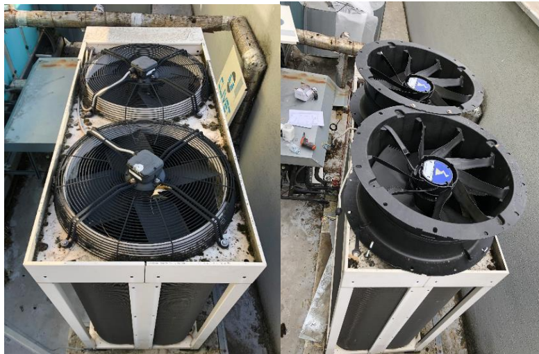
Figure 3 Condensing unit Clivet MSAT 122 on the left with AC fan FB056-8EA 4F.A4P and current regulator according to condensing pressure substituted on the right by EC fan ZN0566ILBDV5P4
