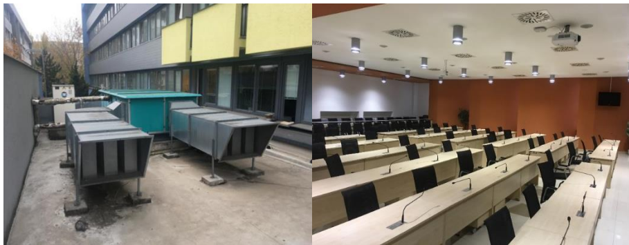
Figure 1 Cooling equipment was a part of ventilation unit, which treated air from conference hall
