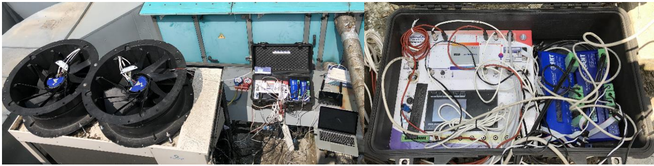
Figure 4 Appliance PA PRO II measured 8 temperatures, two pressures and electric parameters of compressor and condenser fan electric motors with power calculation by two appliances PowerScout
